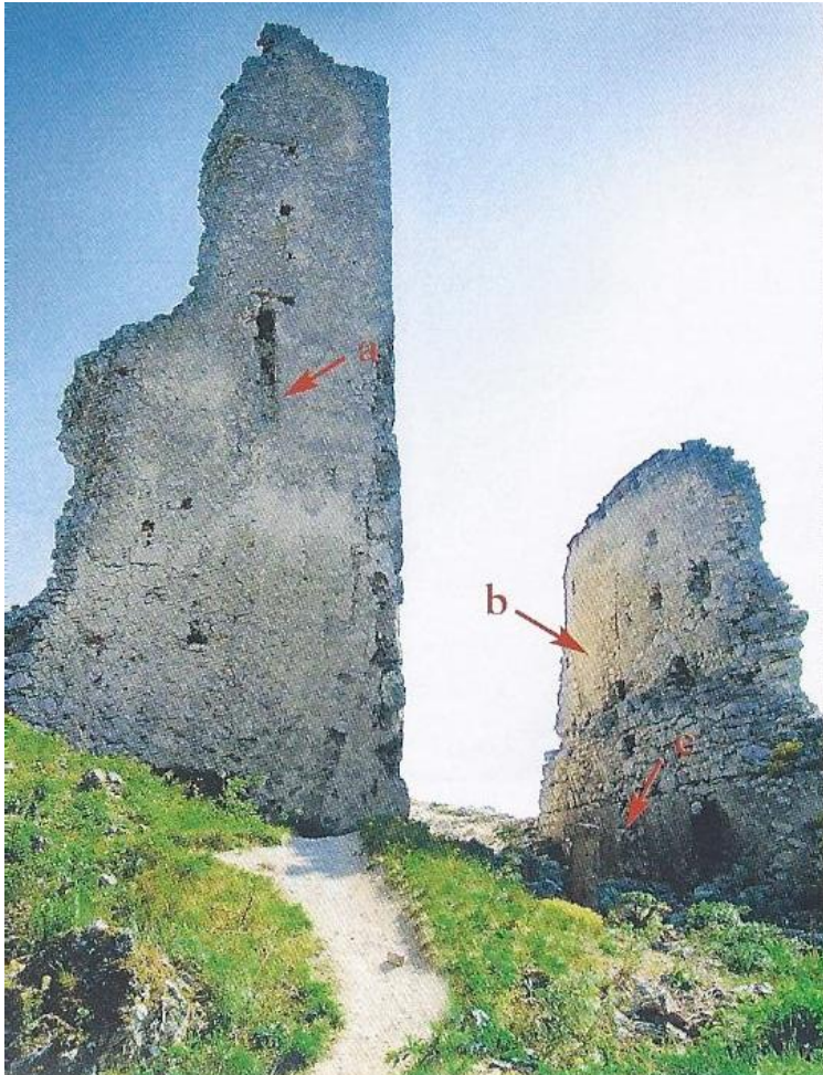
Picture 7 – housing tower and a part of the walls of the upper castle, a – seat of the bearing beam to support the wooden walkway for entering the tower, b – wall extension, c – walled in battlement crenels of the southern wall.
